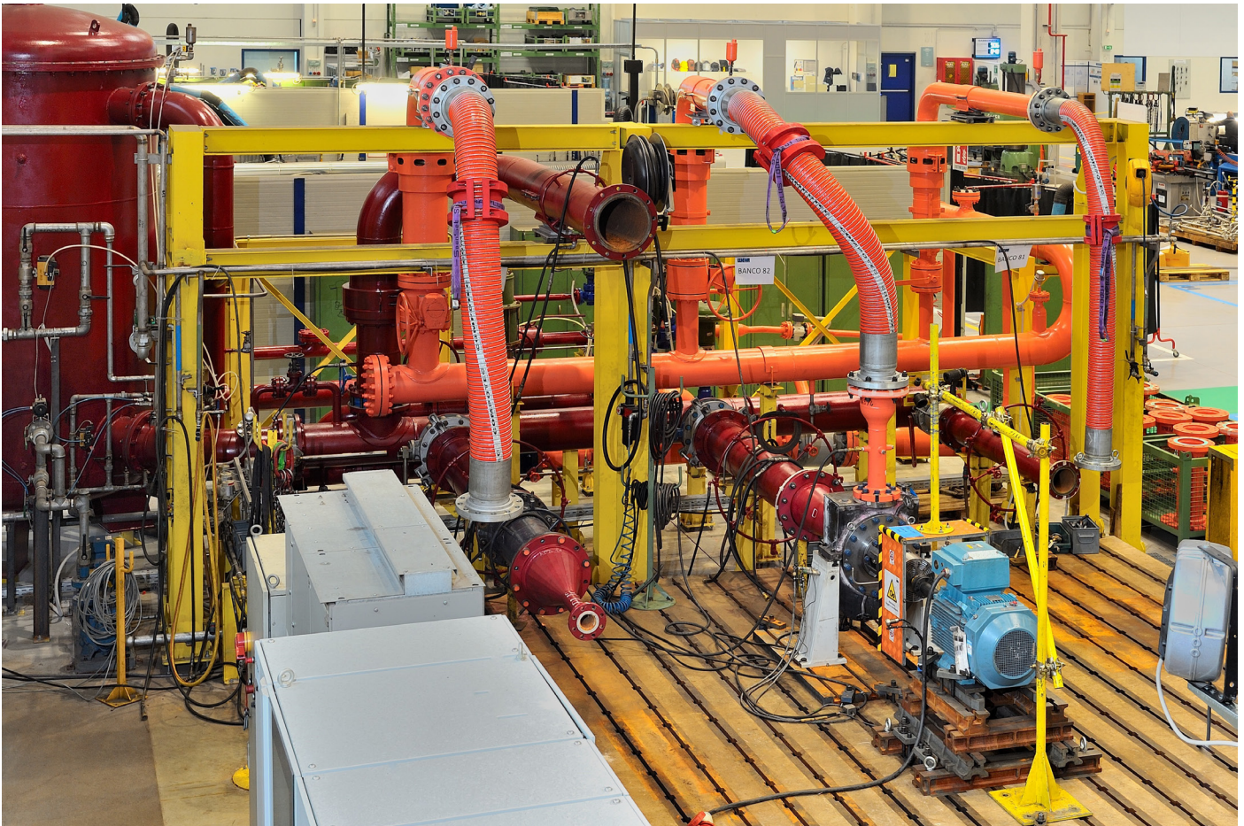
Gabbioneta Test Room – R pumps benches
